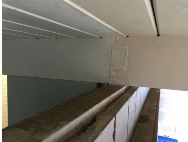
Fig. 6, Out of Plane and Clear Story Opening
